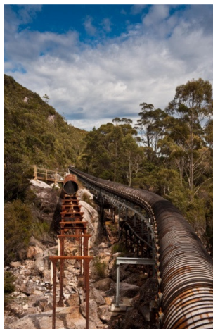
New pipeline at right, with remnant of old pipeline at left. Photography: Hydro Tasmania
