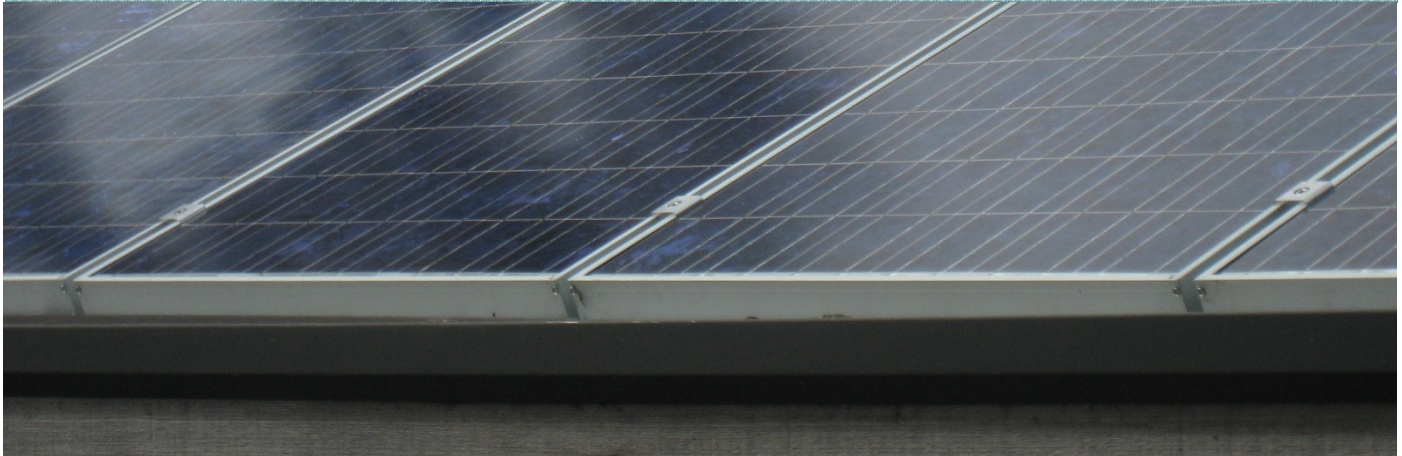
Solar panels on the roof of a heritage building. Photography: Ester Guerzoni
